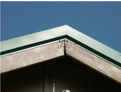
Split fascia at east barn ridge
