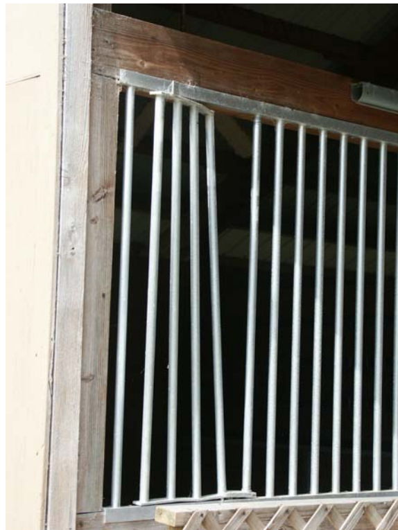
Damaged stall grates at barn
