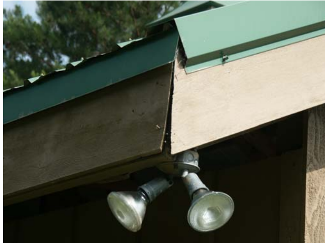
Loose fascia board (SE corner of barn)
