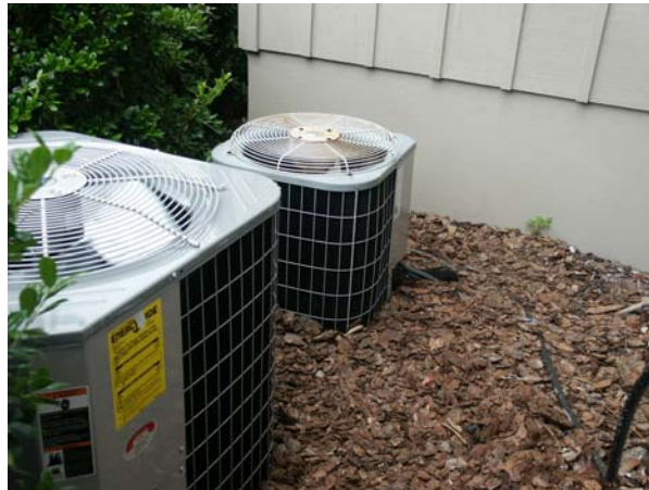
Exterior heat pump units on south end of house
