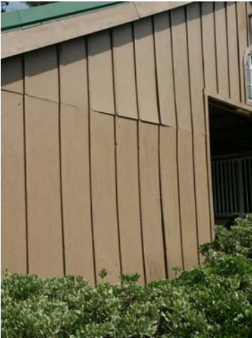
Loose siding (East side of barn)
