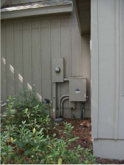
Electric Service and meter at North side of house
