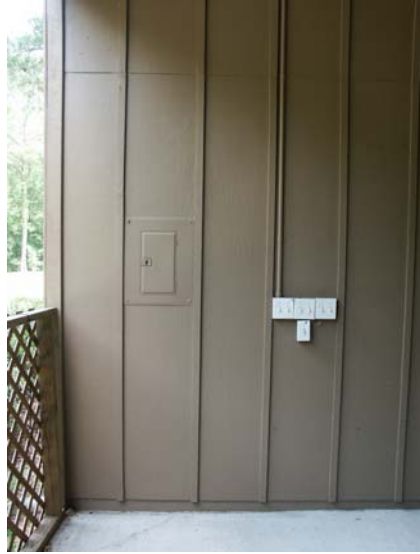
Electric subpanel at barn
