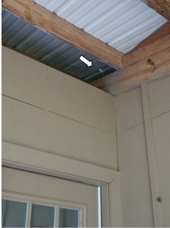
Hole in metal roof at barn
