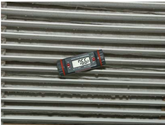
Return air at 76.6 Degrees
