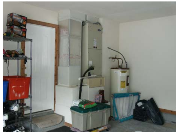
Water Heater in garage. Air handling unit for the lower floor is to left
