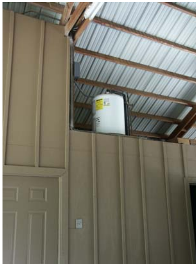
Water Heater above tack room
