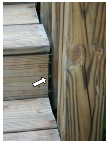
Loose balusters at rear deck rail.
